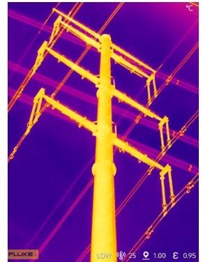
Power transmission lines
